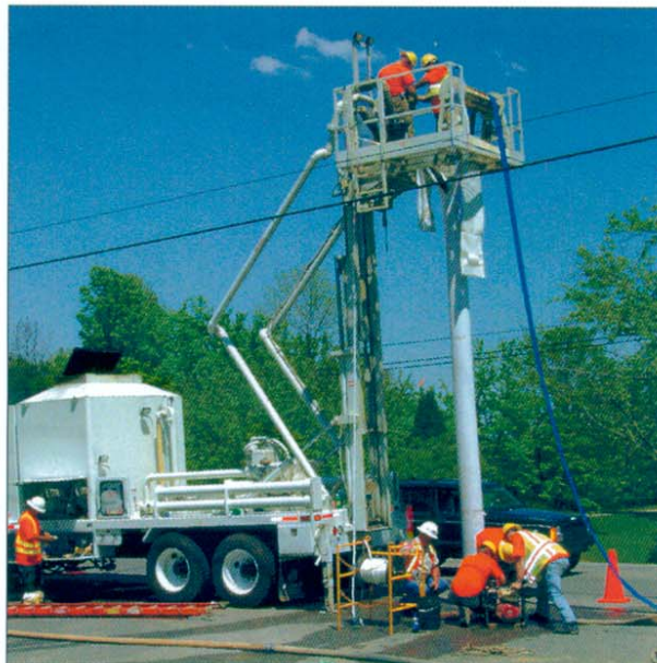
The largest, single wastewater pipeline rehabilitation project in Indiana's history was completed this fall in the City of Madison.
